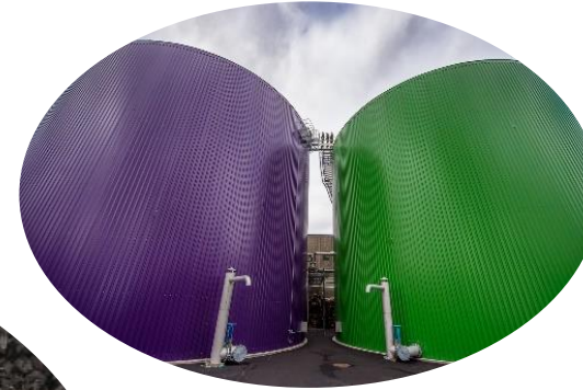
Biogas booster in anaerobic digester
